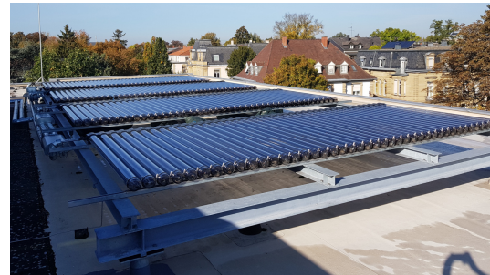
Vacuum tube collectors (roof)
