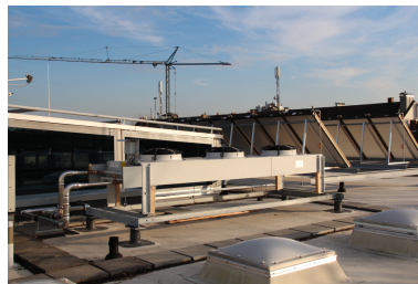
Recooling unit (roof)
